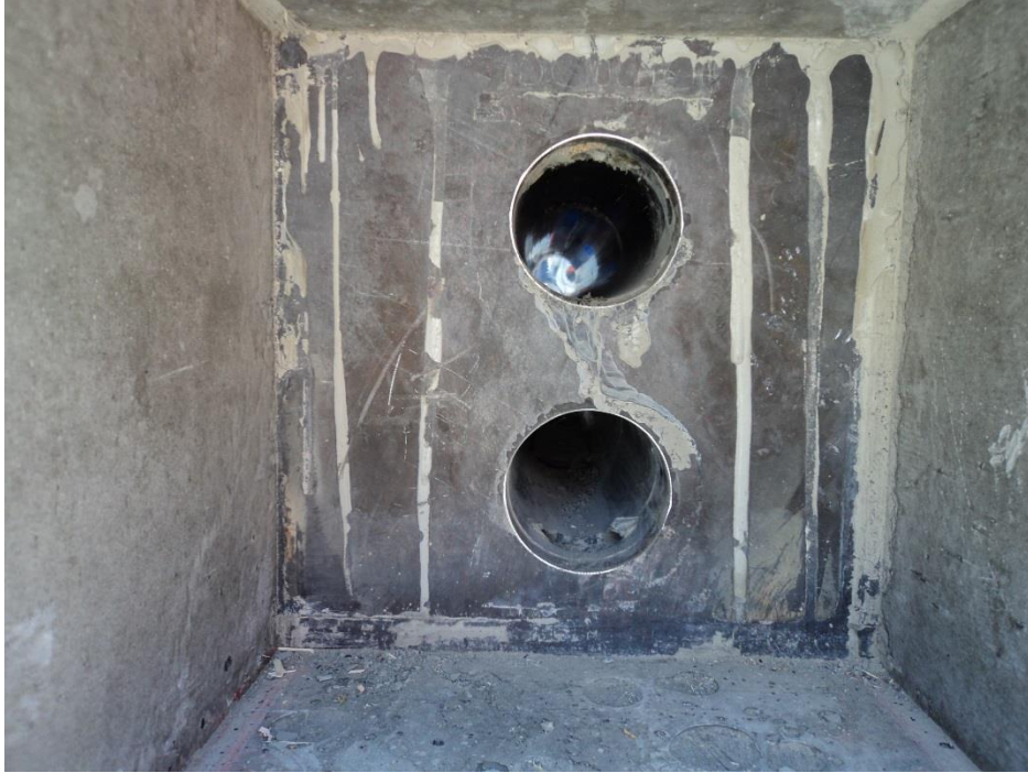
Holes left inside the column
