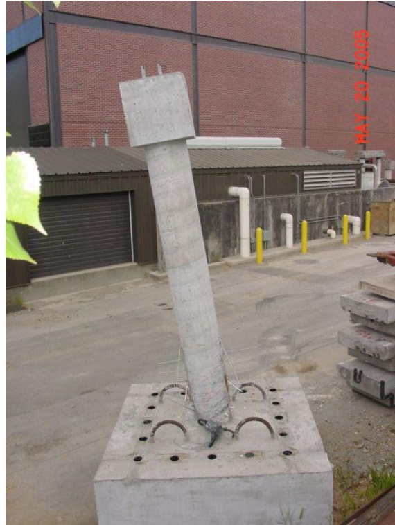
A permanently tilted bridge column
