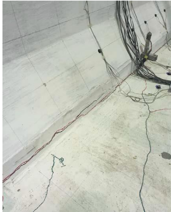
Figure 21 Crack at barrier and deck interface during Test 2
