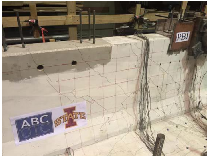
Figure 23 Diagonal cracks during Test 3
