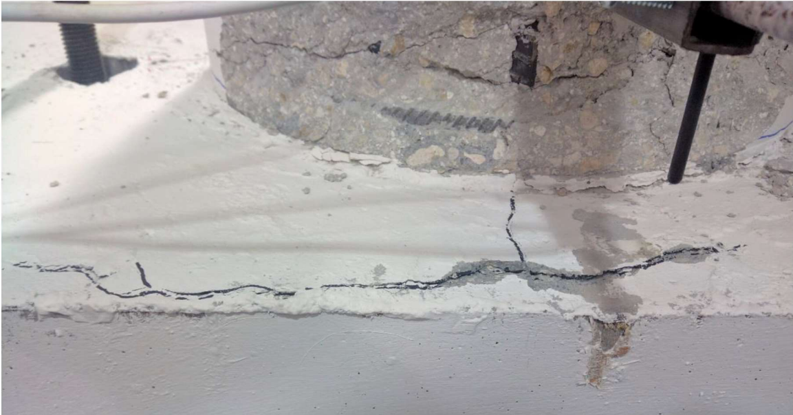
Figure 4-6 Cracks on cap-beam at 4\Delta_y (south).
