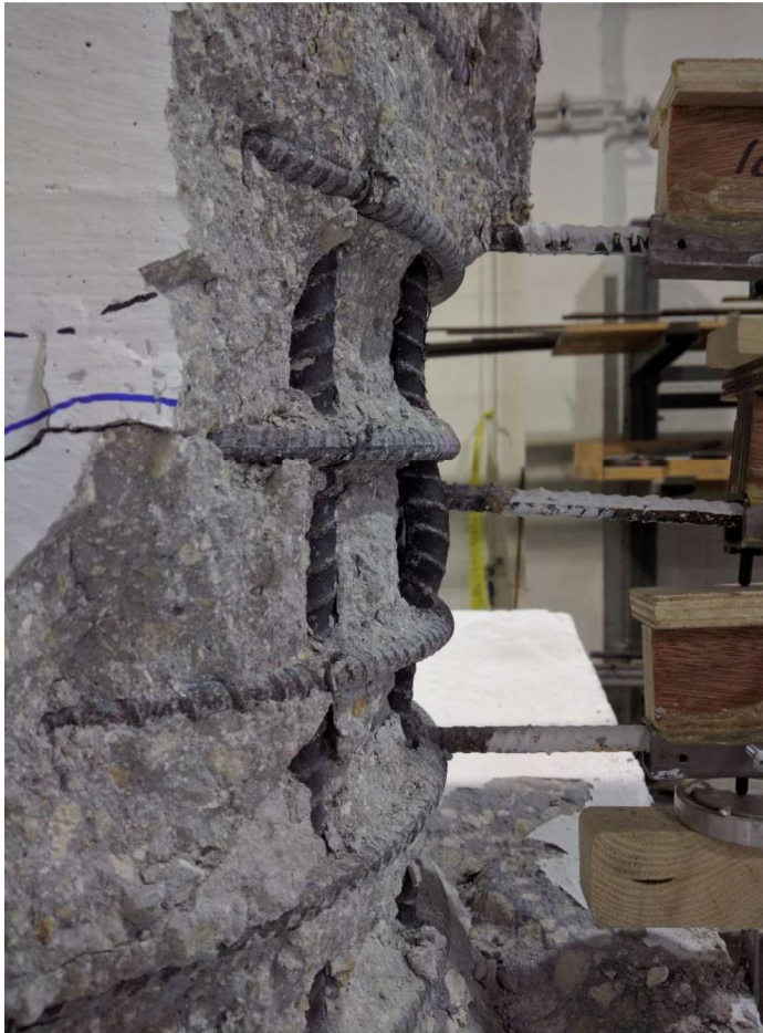
Figure 4-11 First buckling in column longitudinal bars at 6\Delta_y (south).
