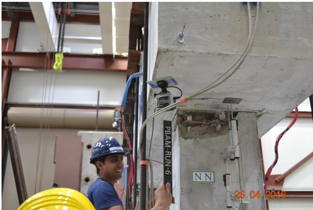
Figure 40. Damage state of ECC plastic hinge and pocket connection under 150% design motion
