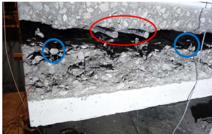
Figure 25 Separation of Top Deck Reinforcement during Testing
