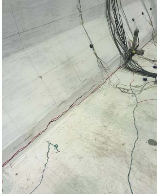
Figure 22 Crack at barrier and deck interface during Test 2
