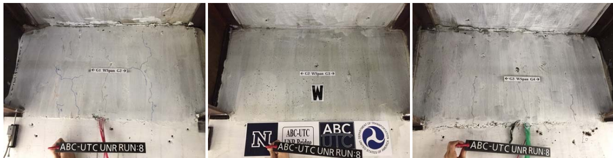
Fig. 69 - Cap beam to girder connection damage state (Images by Elmira Shoushtari)
