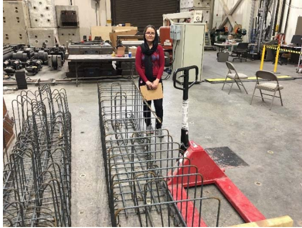
Fig. 44 – Cap beam reinforcement cage
