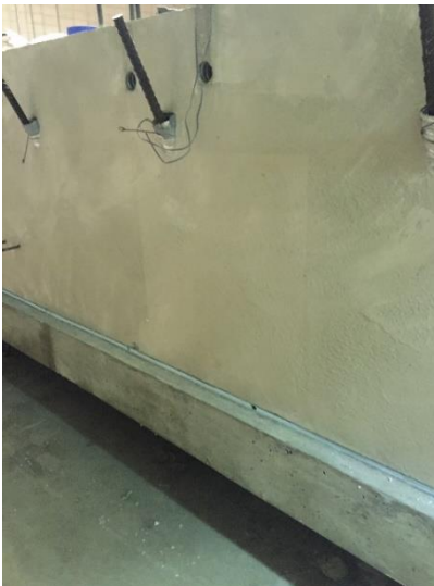
Figure 4.21. Foam added to grout pad to minimize damage cover concrete
