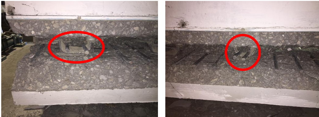
Figure 5.41. Top mat of the bridge deck reinforcement after the Test 6 pull test
