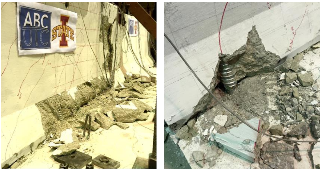
Figure 5.36. Concrete spalling on front of PBI at deck interface and barrier-to-deck connection
