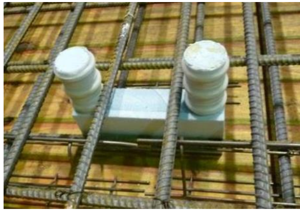
Figure 4.11. U-bar access blocks out with terminated bottom deck steel and top deck steel positioned to be within a U-bar connection
