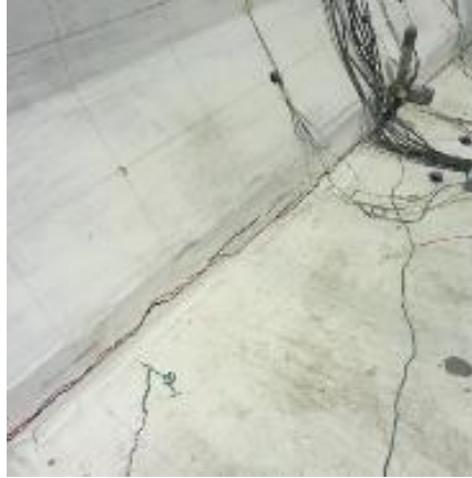
Figure 5.12. Crack at the barrier-to-deck interface in PBU during Test 2
