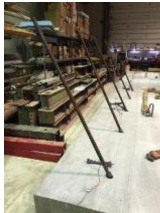
Figure 4.14. Inclined reinforcing bars connected to bridge deck before placement of precast barrier
