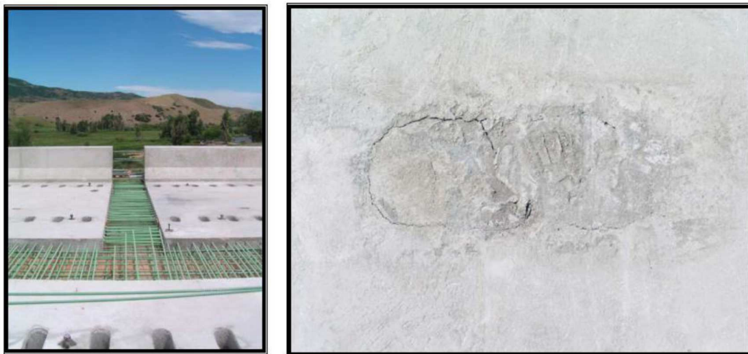
Figure 9: Shrinkage crack in the blockout type of ABC closure joint [13]
