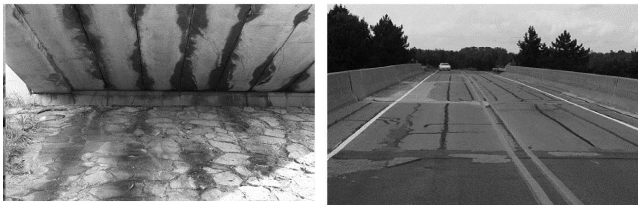
Figure 10: Longitude deck cracking of ABC closure joint [14]
