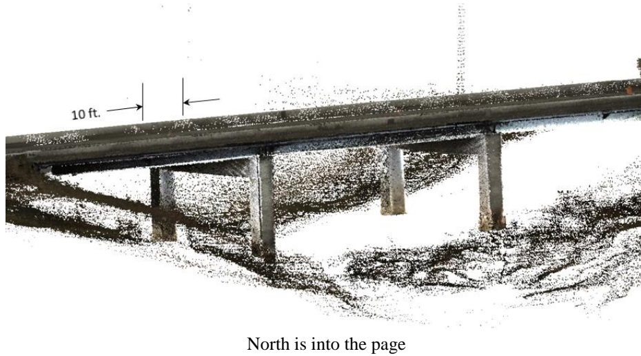
Figure 7. Full view at deck level of Keg Creek Bridge including bridge deck and ground features
