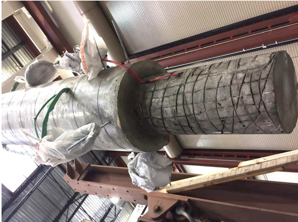
Figure A.36 Precast cap beam reinforcement cage
