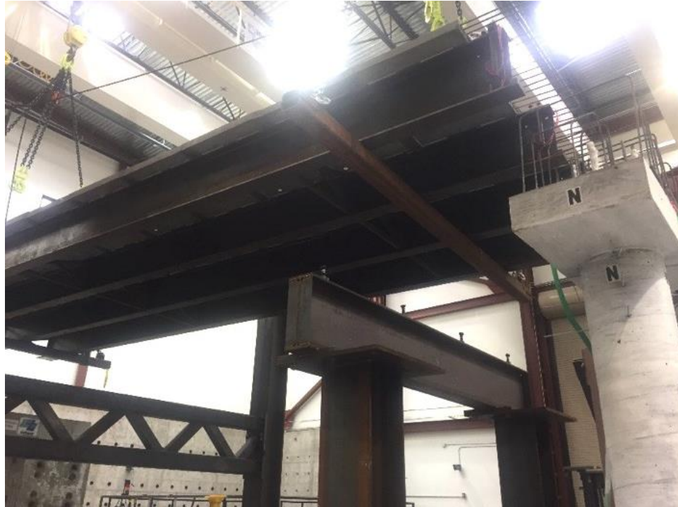
Figure A.49 Placement of east span over the abutment seat and precast cap beam
