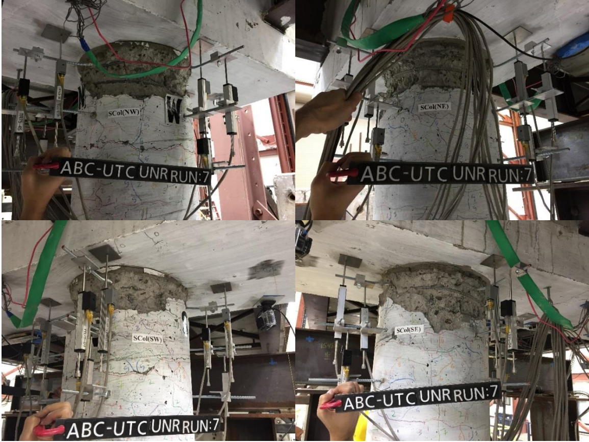
Figure B.8 Damage states of the south column plastic hinges after Run 7
