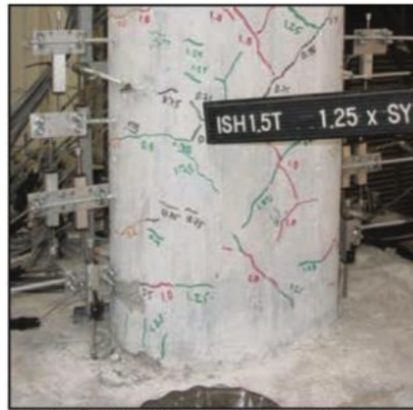
DS-2: first spalling and shear cracks
