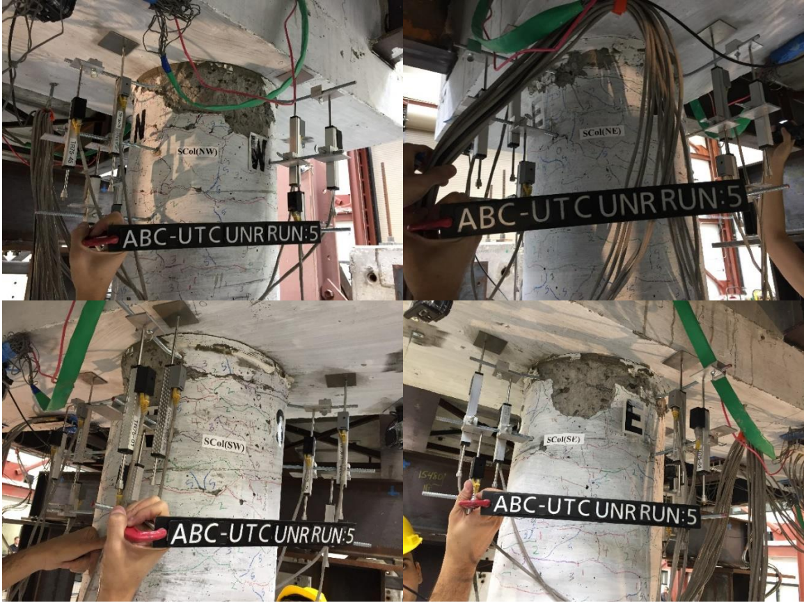
Figure B.6 Damage states of the south column plastic hinges after Run 5
