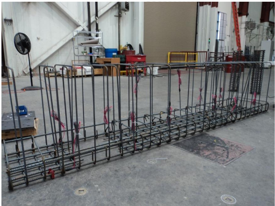
Figure A.37 Precast cap beam reinforcement cage
