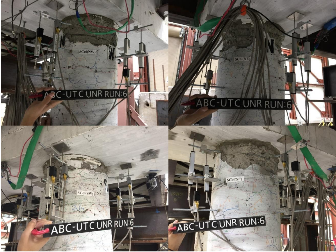
Figure B.7 Damage states of the south column plastic hinges after Run 6
