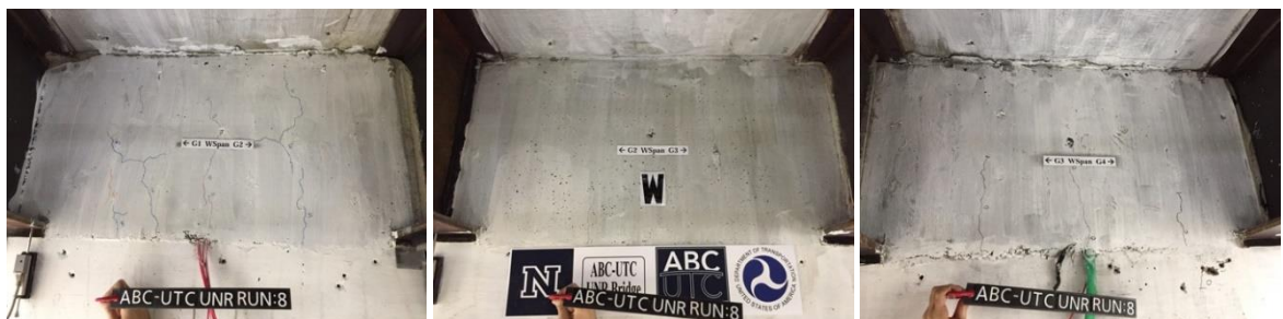
Figure 3.20 Cap beam to girder connection damage state (Images by Elmira Shoushtari)
