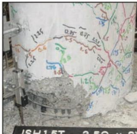
DS-5: imminent failure
