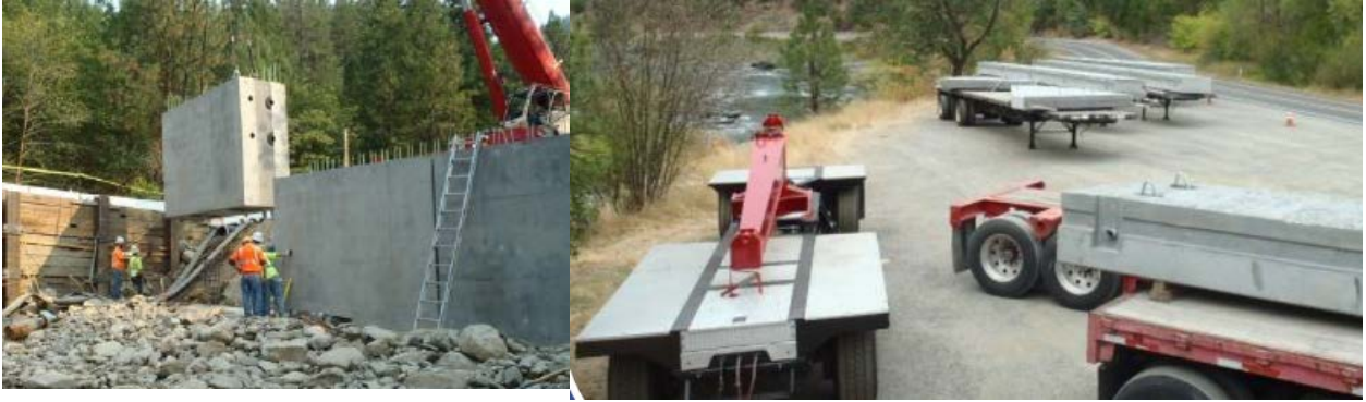
Fig. 4 – Wingwalss and abutment assembly (left) and deck precast segments (right) for Fort Goff Creek bridge in California (photos are courtesy of Dorie Mellon as adopted from Caltrans ABC-UTC seminar)
