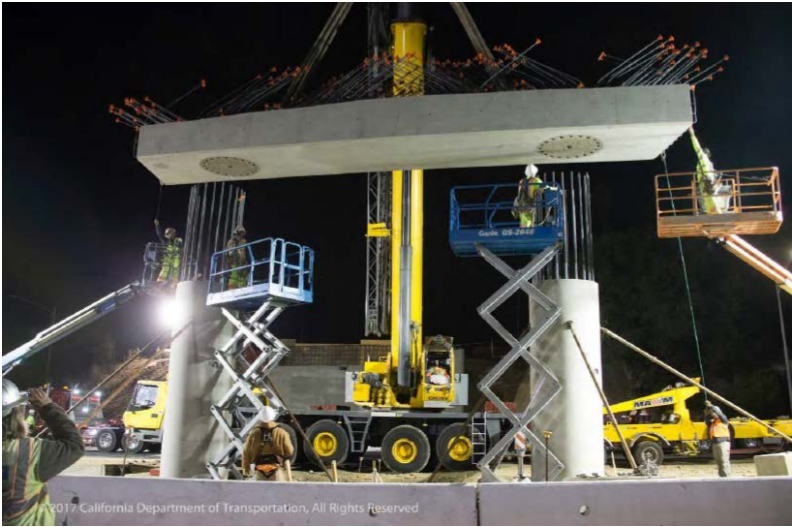
Fig. 5 – Precast columns and drop bent cap for Laurel Street Overcrossing project in California (photos are courtesy of Dorie Mellon as adopted from Caltrans ABC-UTC seminar)
