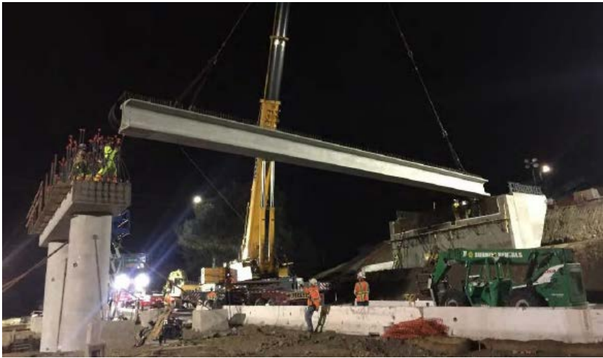
Fig. 6 – Installing a precast girder for Laurel Street Overcrossing project in California (photos are courtesy of Dorie Mellon as adopted from Caltrans ABC-UTC seminar)
