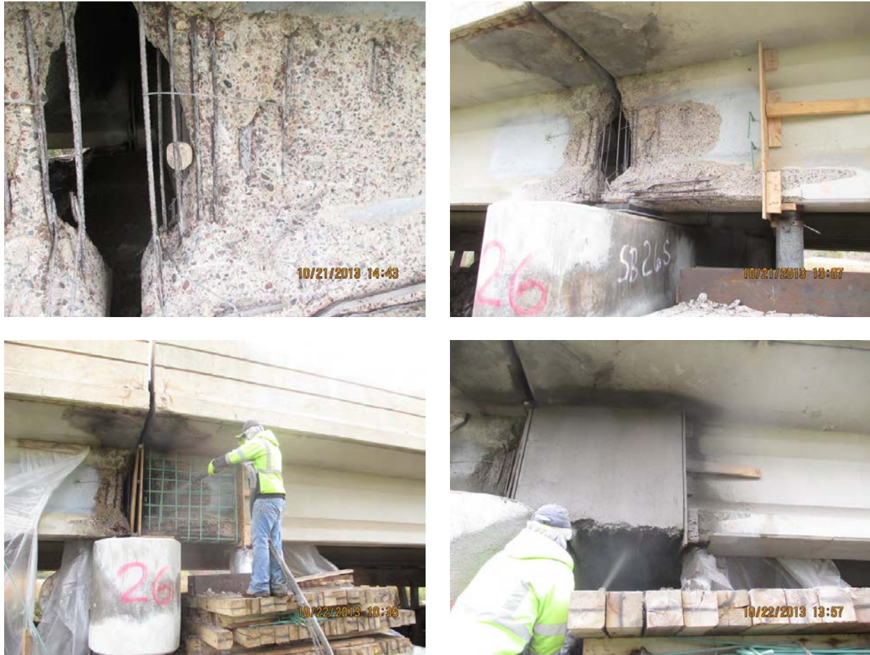
Figure 1. Reinforced shotcrete repair of prestressed bridge girder ends in Minnesota (Photos adopted from Shield 2018)
