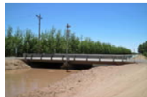
NM 186 crossing the La Union Canal in Anthony, New Mexico Courtesy of New Mexico State University
