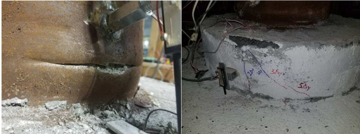
Figure 13. Ductile tearing of the CFT (left), and crack pattern in UHPC step (right)
