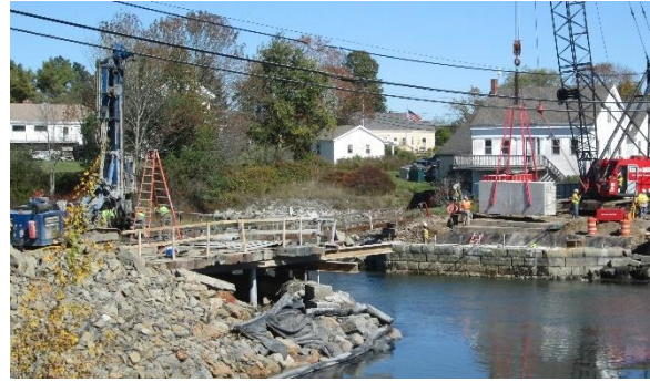
Figure 2 - Drilling of Spun Pipe Piles at Near Abutment while Precast Abutment Pieces Placed at Far Side
