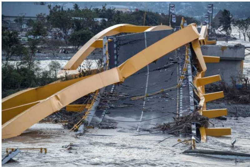
Figure 1. Ponulele Bridge Destroyed by 2018 Tsunami
