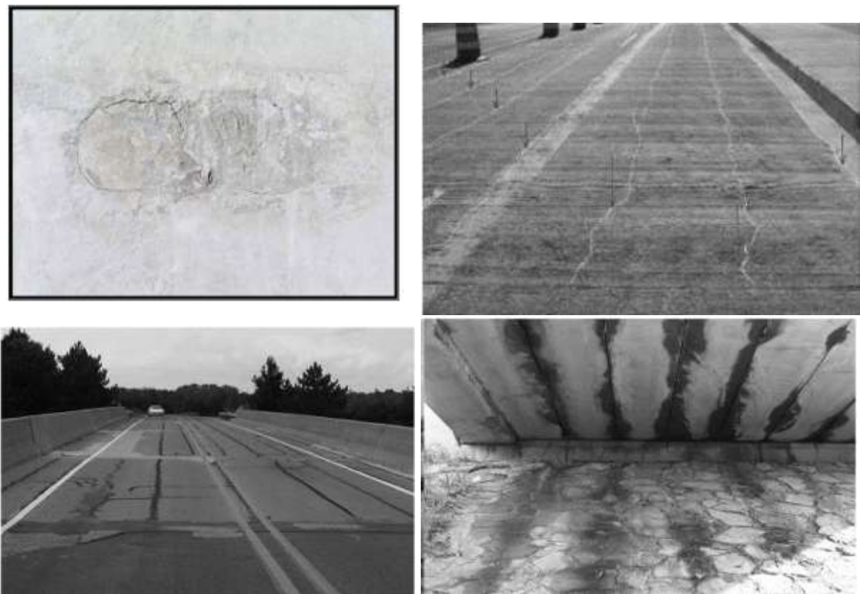
Figure 1: Examples of defects in ABC closure joints; shrinkage due to the excess water in concrete (left) [1], and longitudinal deck cracking of ABC closure joint (right) [2].
