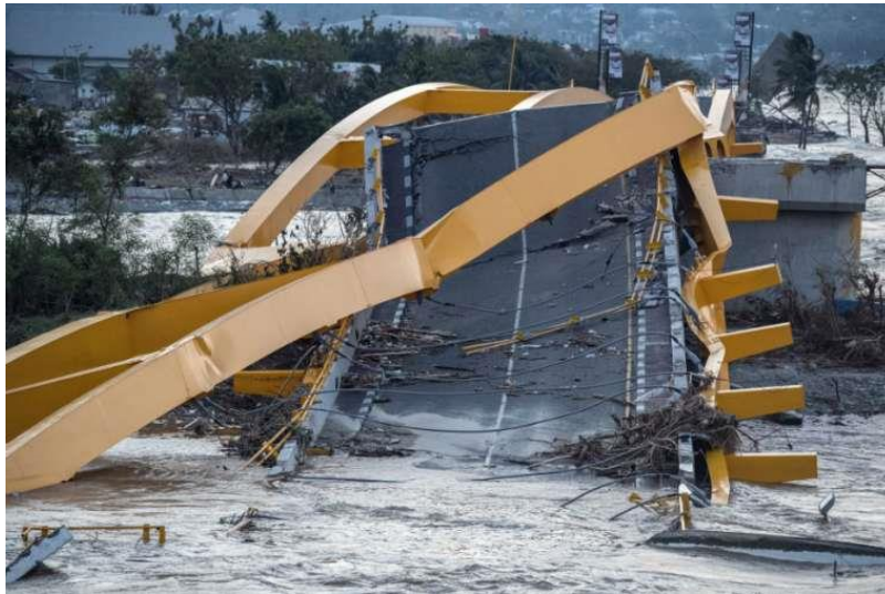
Figure 1. Ponulele Bridge Destroyed by 2018 Tsunami
