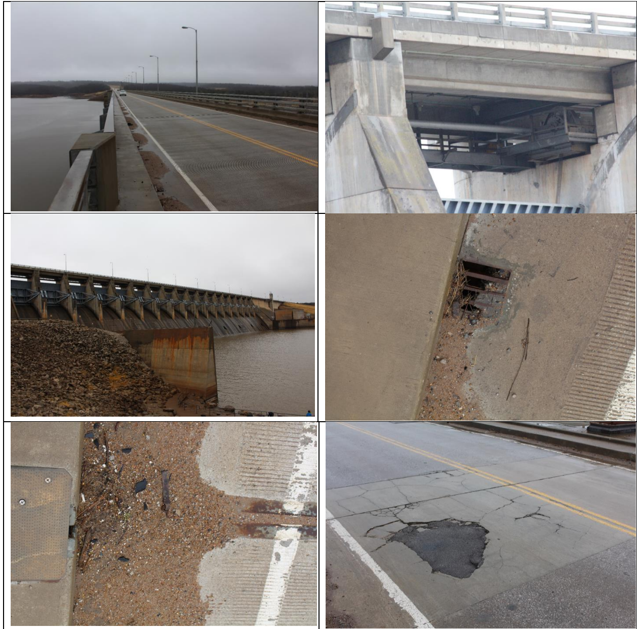
Figure 2 - Prefabricated Bridge Elements and Systems (PBES) – Selected Photographs of Bridge over Keystone Lake Spillway.
