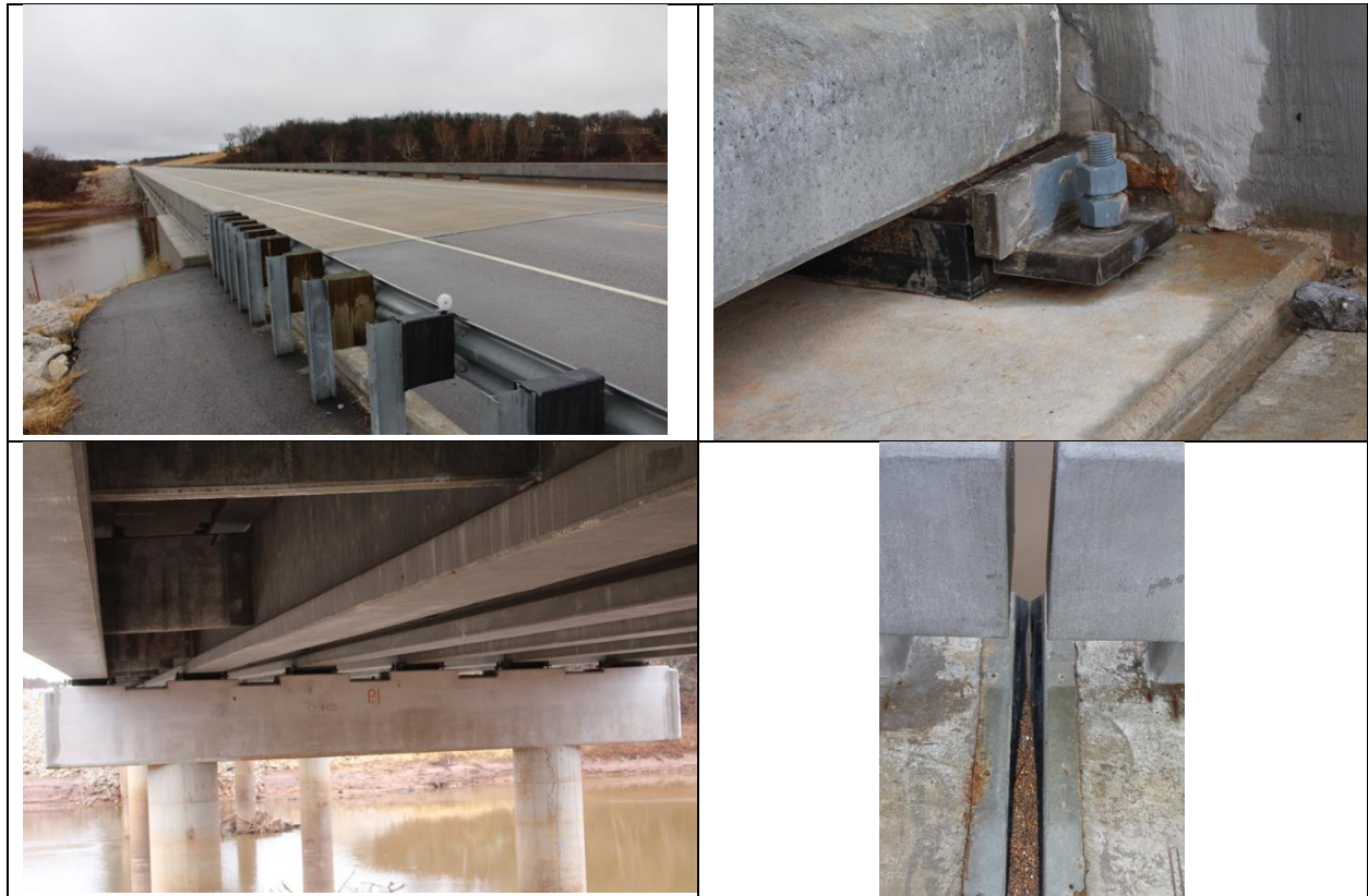
Figure 1 - Slide-In Bridge Construction (SIBC) –Selected Photographs of Bridge over Cottonwood creek on state highway 51, just west of SH-48.
