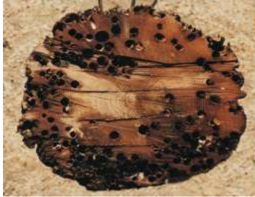
Figure 3: Tunneling in a timber pile caused by Teredo and Bankia (M. Iskander, 2003)
