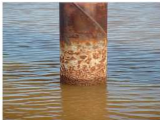
Figure 4: Corrosion in steel pile
