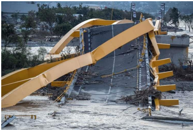
Figure 1. Ponulele Bridge Destroyed by 2018 Tsunami
