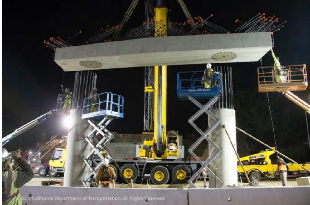
Fig. 4 – Precast columns and drop bent cap for Laurel Street Overcrossing project in California (photos are courtesy of Dorie Mellon as adopted from Caltrans ABC-UTC seminar)
