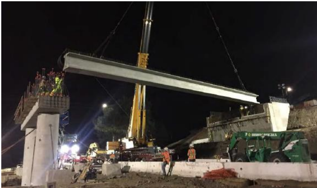
Fig. 5 – Installing a precast girder for Laurel Street Overcrossing project in California (photos are courtesy of Dorie Mellon as adopted from Caltrans ABC-UTC seminar)
