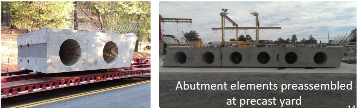
Fig. 2 – Precast abutment segments for Fort Goff Creek bridge in California (photos are courtesy of Dorie Mellon as adopted from Caltrans ABC-UTC seminar)
