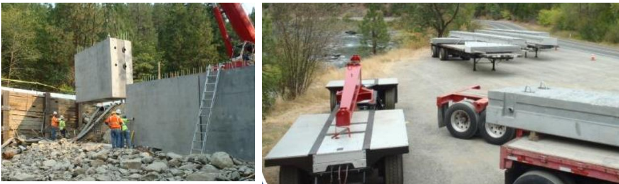
Fig. 3 – Wingwalls and abutment assembly (left) and deck precast segments (right) for Fort Goff Creek bridge in California (photos are courtesy of Dorie Mellon as adopted from Caltrans ABC-UTC seminar)
