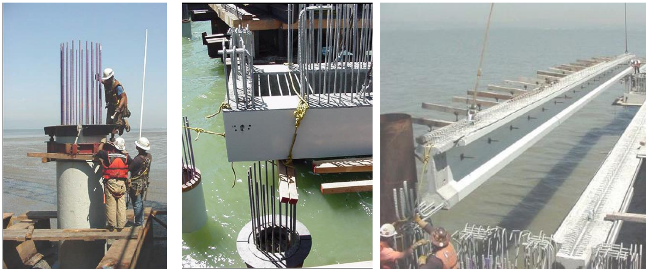
Fig. 1 – San Mateo-Hayward Bridge Widening Project in California using prefabricated elements (courtesy of Caltrans ABC pilot program, Roberto Lacalle)
