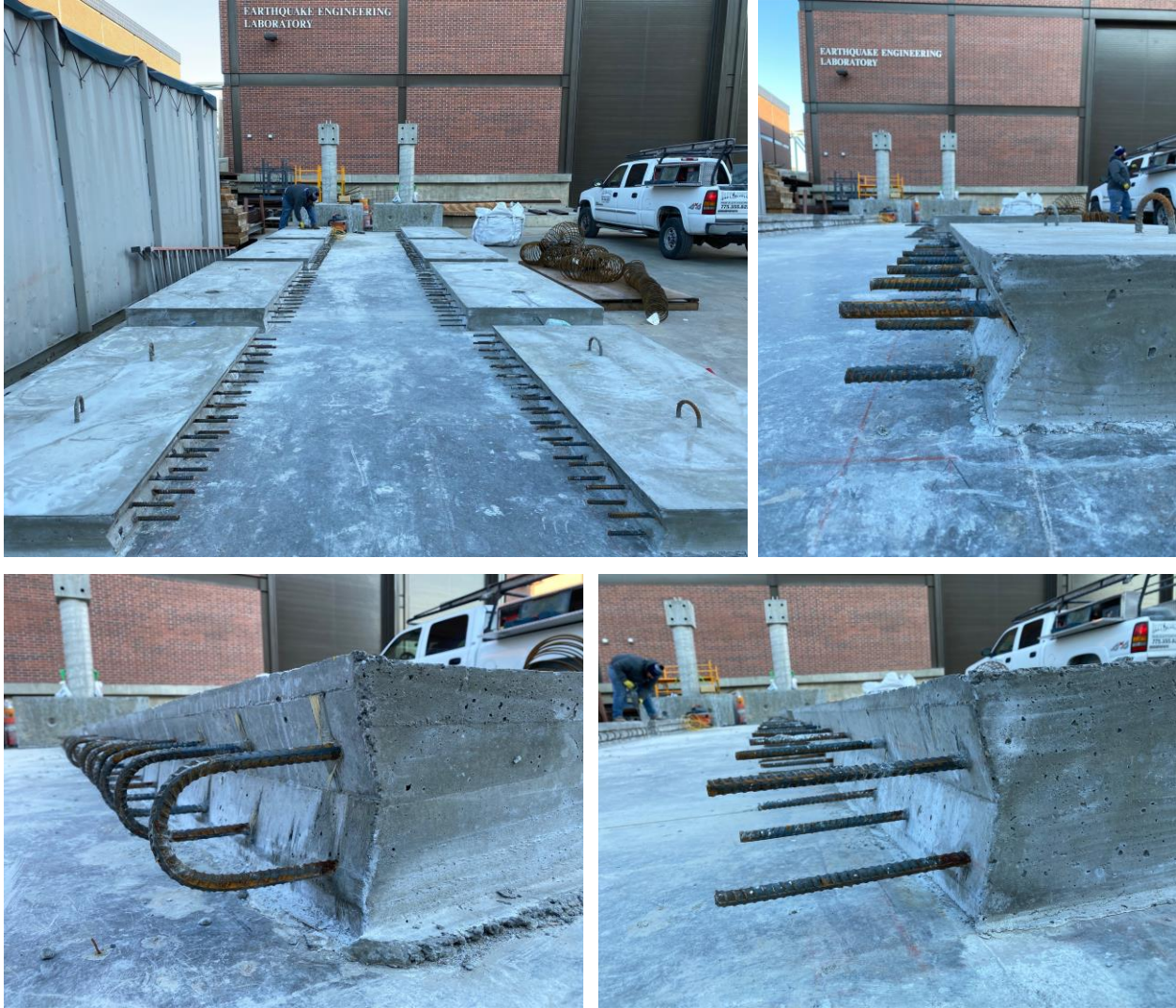
Figure 20 – Close-up views of the constructed deck panels and shear keys for the field joints.
