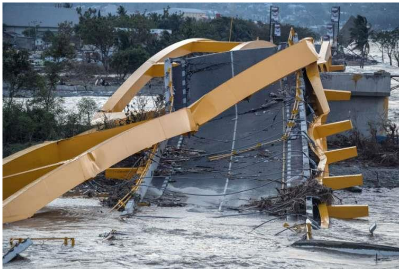
Figure 1. Ponulele Bridge Destroyed by 2018 Tsunami
