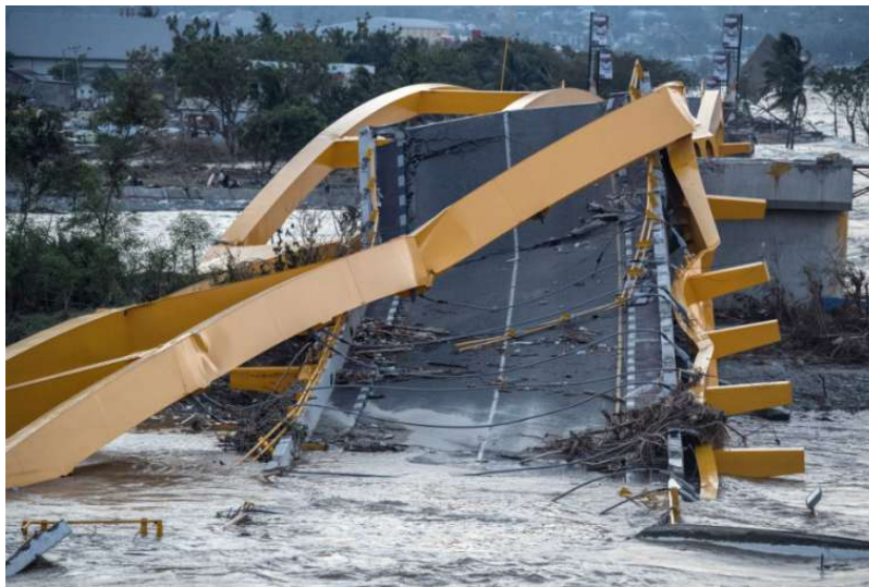
Figure 1. Ponulele Bridge Destroyed by 2018 Tsunami
