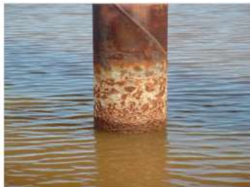
Figure 4: Corrosion in steel pile
