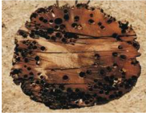
Figure 3: Tunneling in a timber pile caused by Teredo and Bankia (M. Iskander, 2003)
