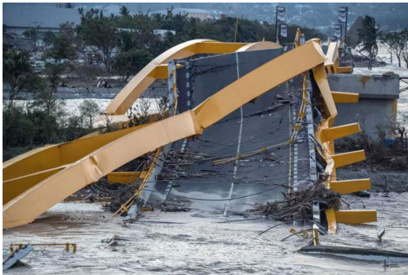
Figure 1. Ponulele Bridge Destroyed by 2018 Tsunami
