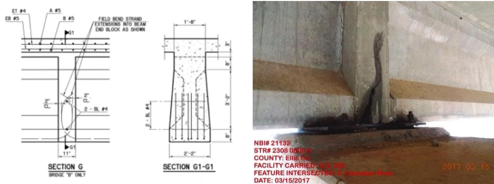
Figure 1. Detail for a typical continuity linkage block used in Oklahoma (left) and photo of a linkage block exhibiting cracking from restraint induced moments (right)
