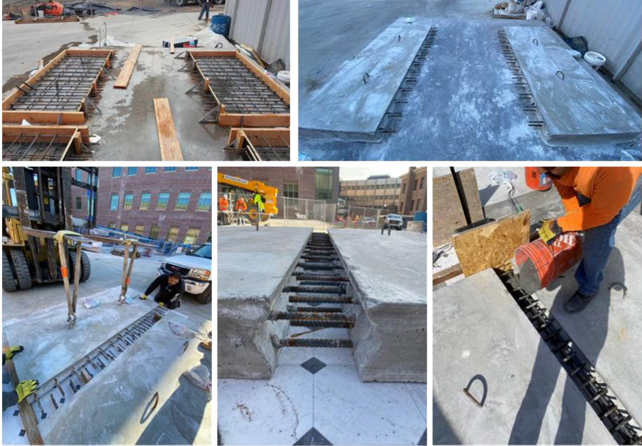
Figure 4-3: Photographs from the fabrication process and illustration of the sequence of constructing test specimens.
