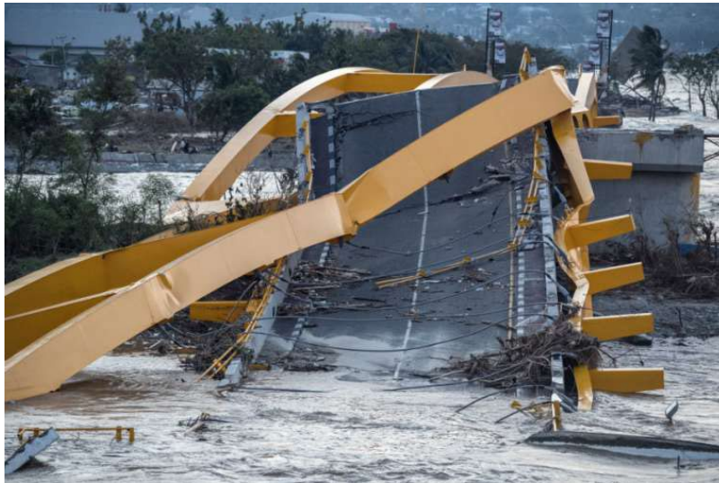
Figure 1. Ponulele Bridge Destroyed by 2018 Tsunami
