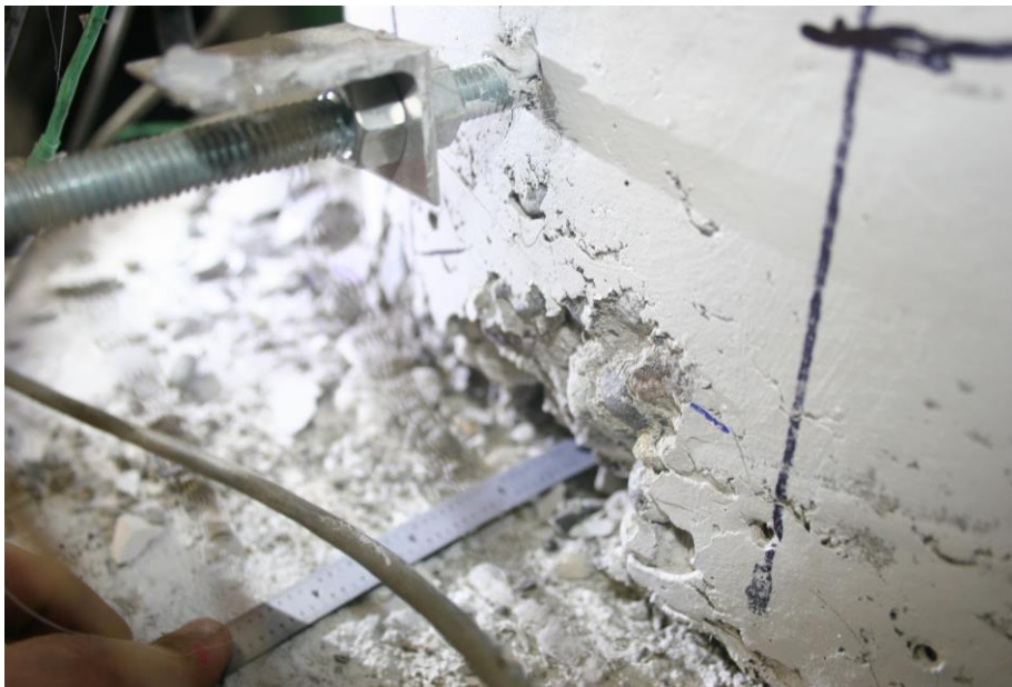
Figure 3.23. Specimen 30-21-R 2 in. Deep Crack at Northern Base of Column at 4.0% Drift
