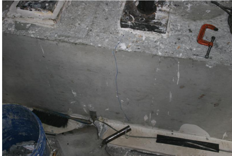
Figure 3.47. Specimen 30-21-LD Crack on Southern Side of Transfer Block
