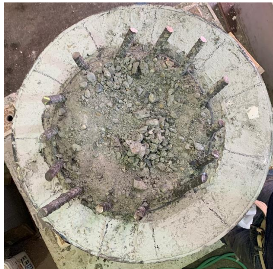
Figure 3.30. Top of Specimen 30-21-R Pile with Column Removed
