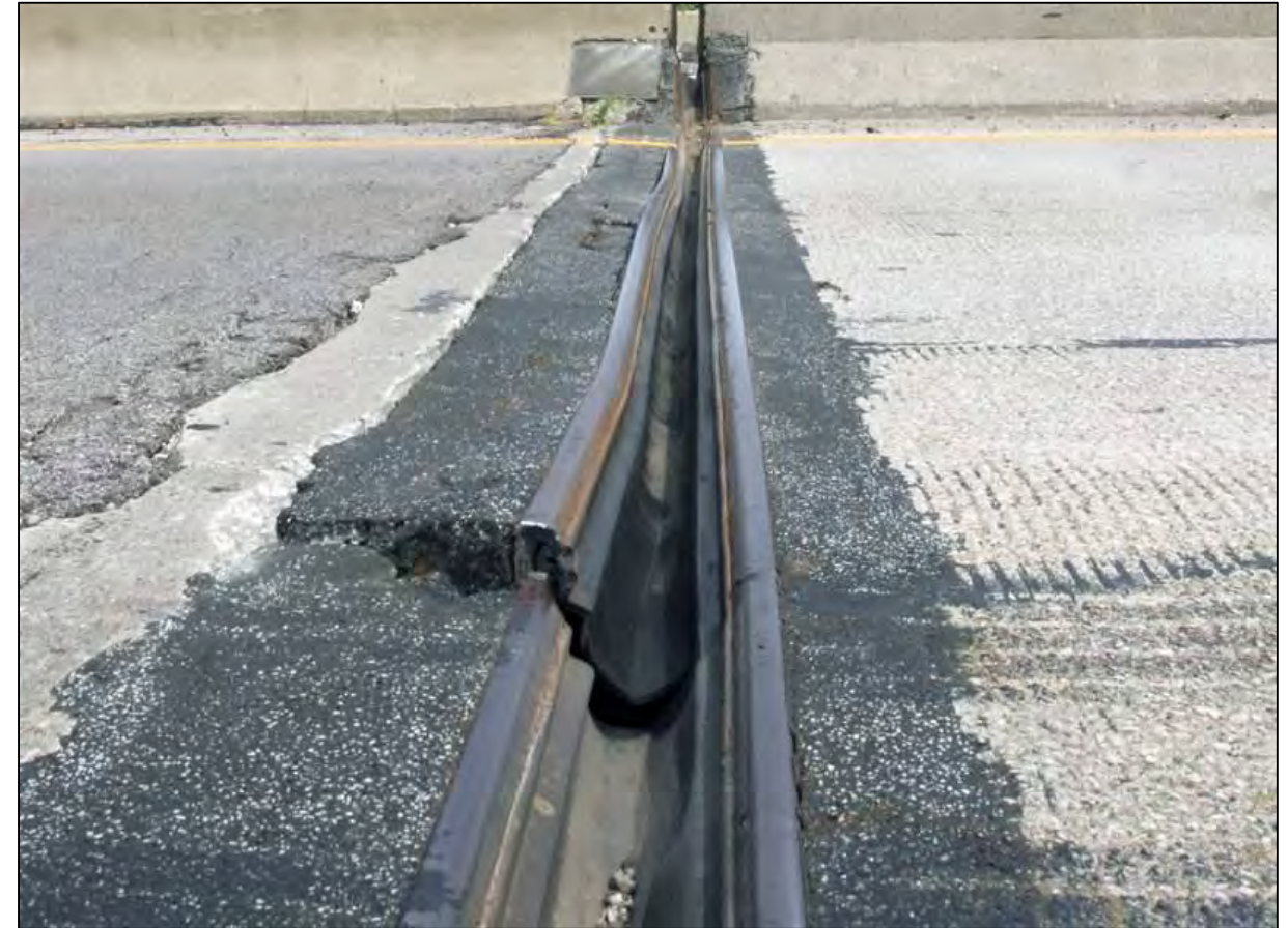
Expansion joint damage ( http://www.toledoblade.com/local/2011/07/08/Defective-bridge-expansion-joint-causes-I-75-delays.html )
