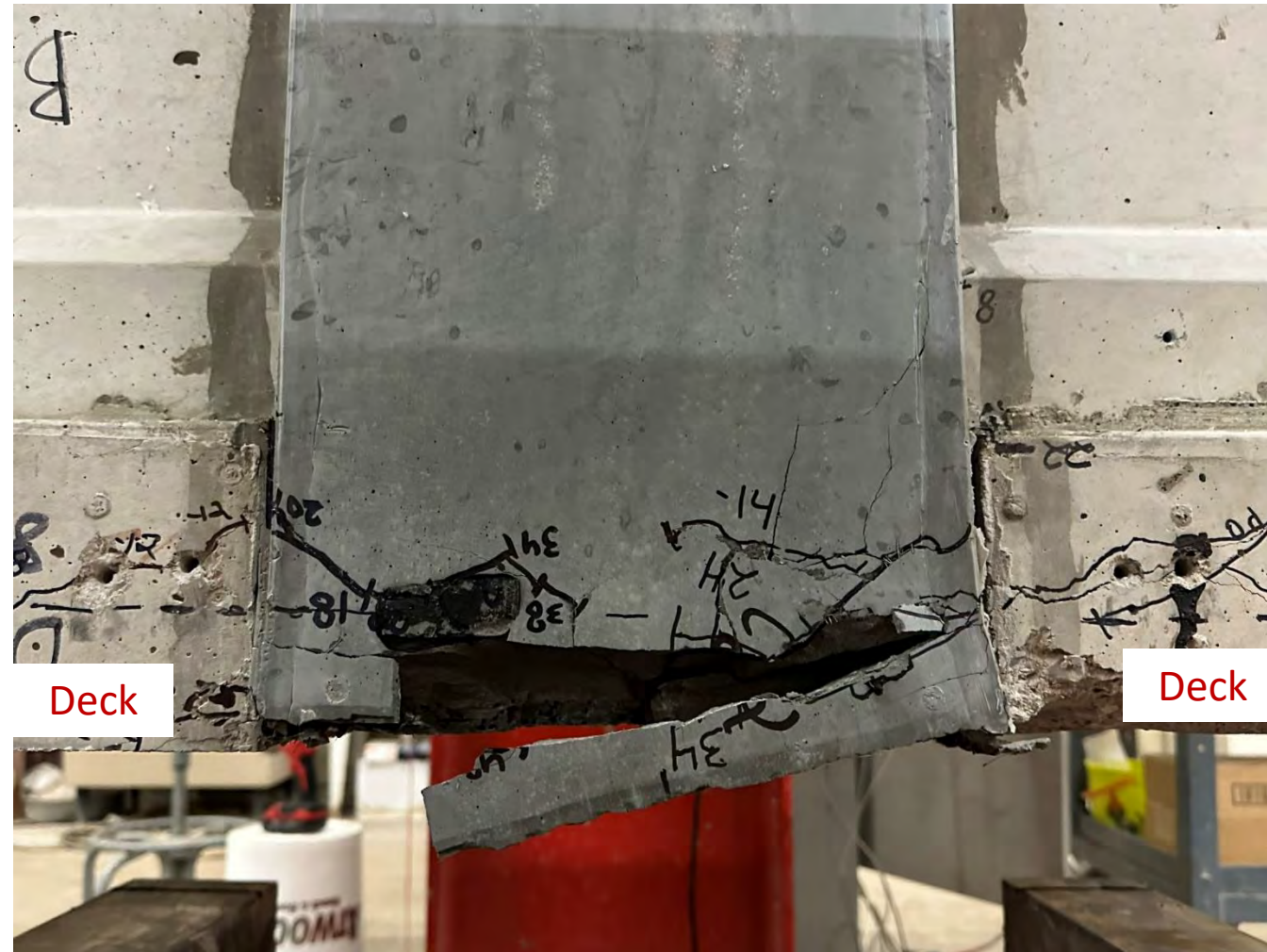
Horizontal cracking and spalling of UHPC with no fibers during negative moment test
