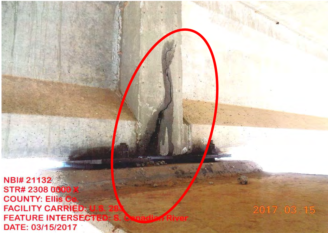
Typical cracking in continuity connection on U.S. 283 over S. Canadian River (Photo courtesy of Walt Peters)
