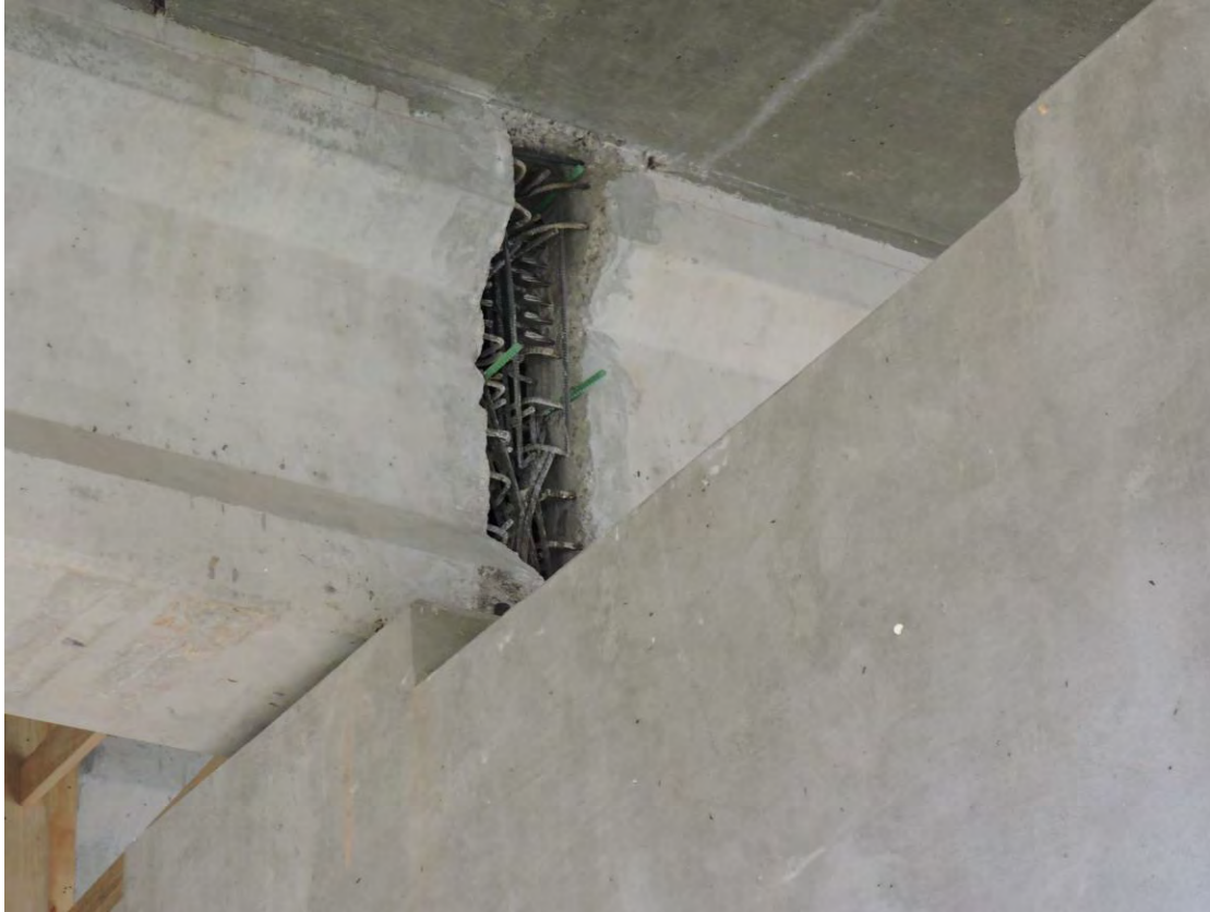
Exposed reinforcement after joint demolition
