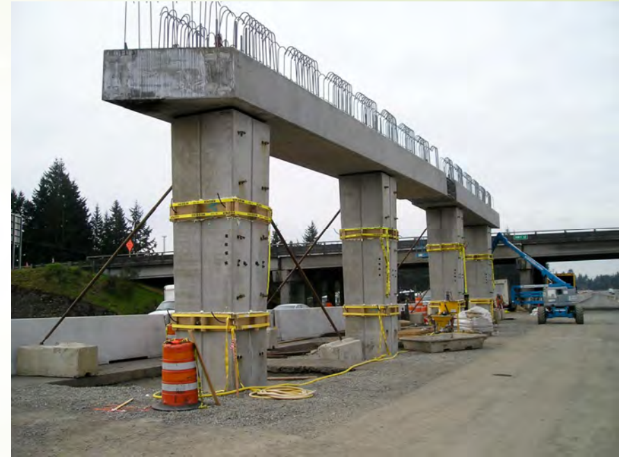
Photo. Grouting the joints between column segments and between columns and cap beam.
