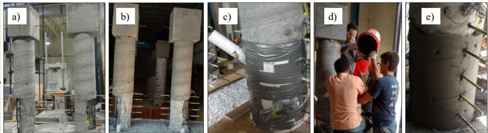
Figure - Repair Procedure: a) damaged part before repair, b) damaged part after sandblasting treatment, c) formwork for the repair plastering, d) casting UHPC, and e) damaged part after repair.
