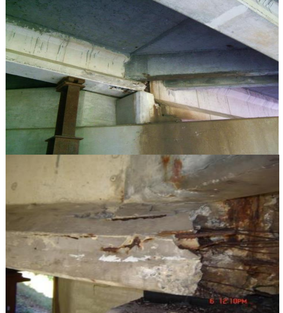
Beam End Deterioration
