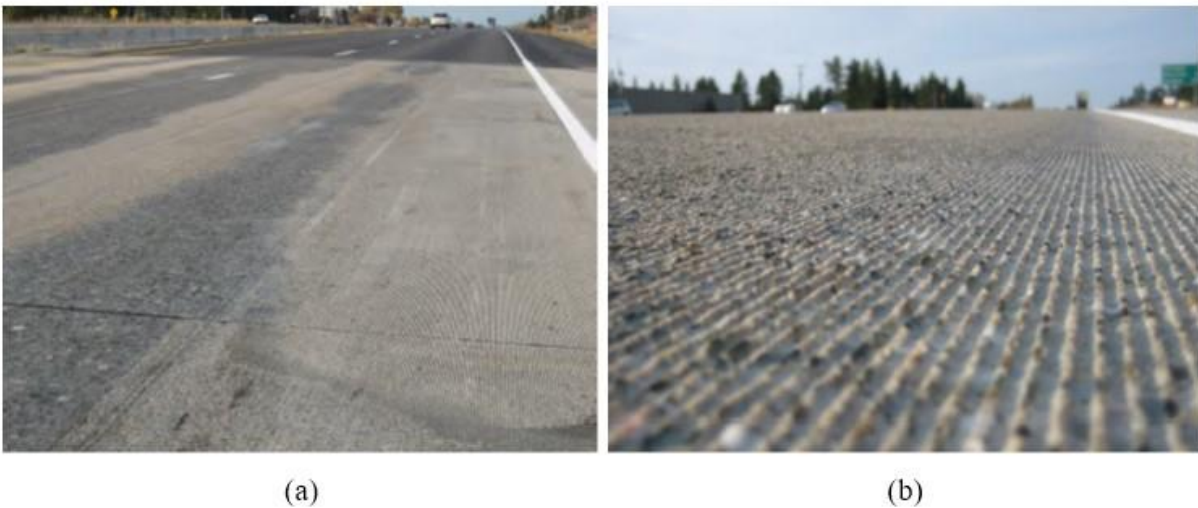
Figure 1-3. (a) Wheel path PPC inlay, (b) PPC overlay with diamond grinding (Anderson et al. 2013)
