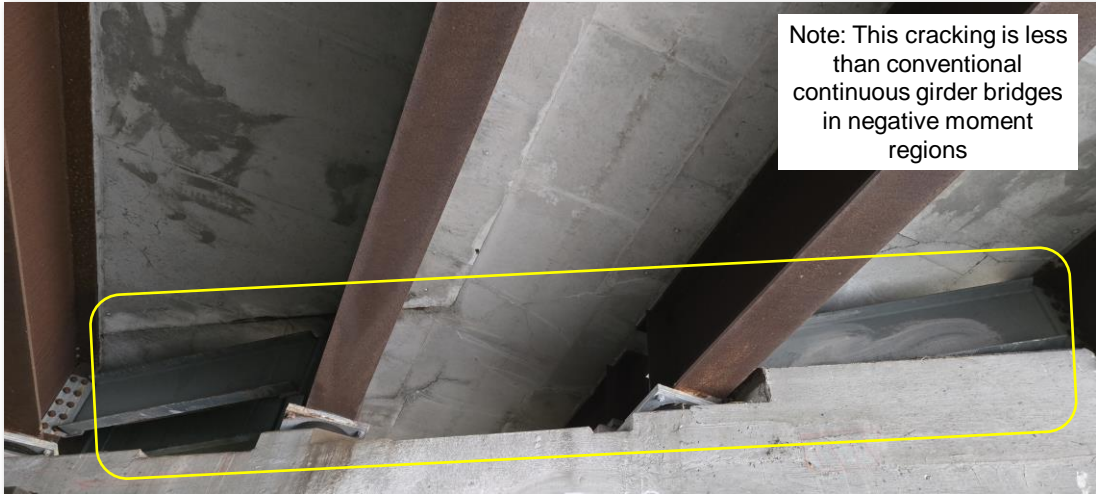
Link slabs in 2024 - 13 years in service
