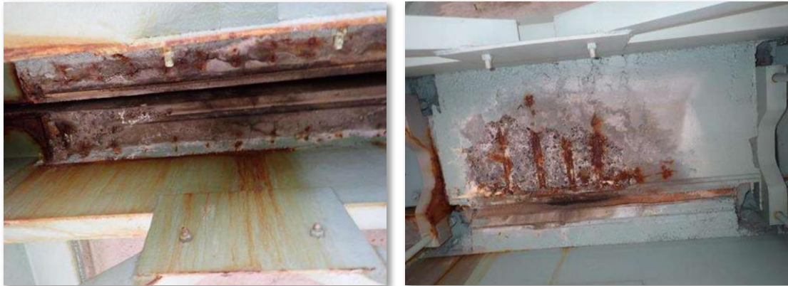
2023 Condition 33 years in service CIP closure pours at leaking deck expansion joints
