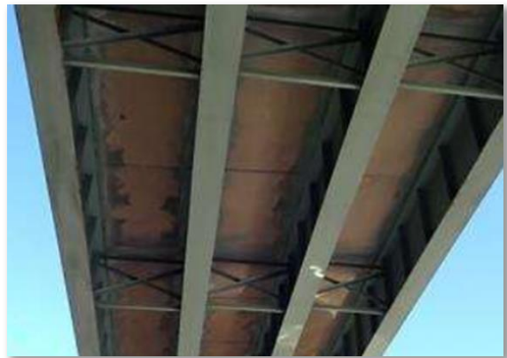
2023 Condition 33 years in service
