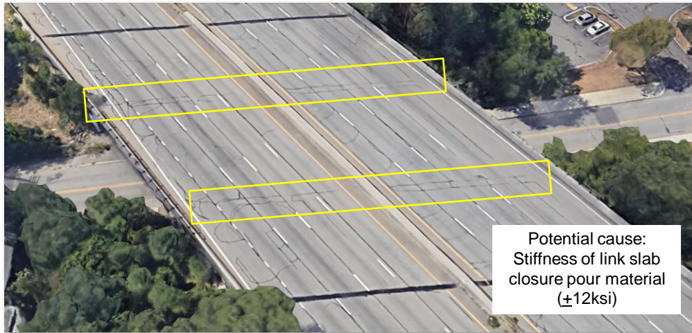
Overlay in 2024 - 13 years in service Minor cracking at link slabs ( not leaking )
