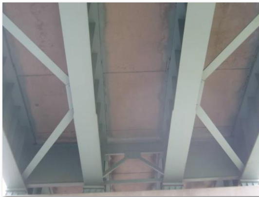
2010 Condition 20 years in service
