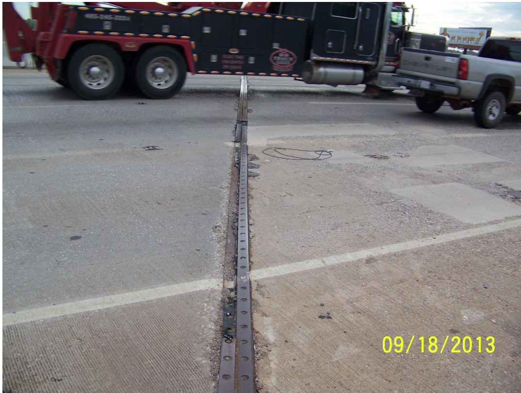
Bridge Expansion Joint with Damage to Steel Armoring (Photo courtesy of Walt Peters, ODOT)
