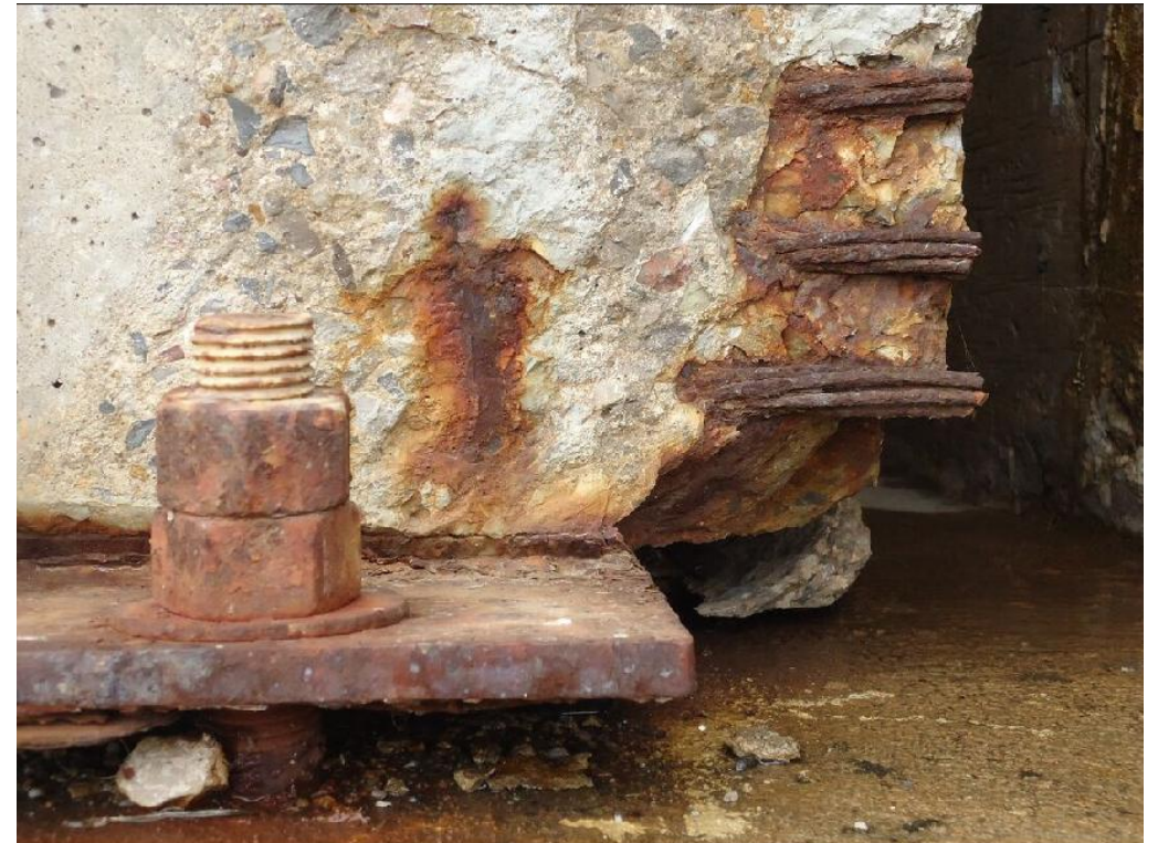
Spalling Around Prestressing Strand Ends in In-Service Prestressed Concrete Girder (Photo by Royce Floyd)
