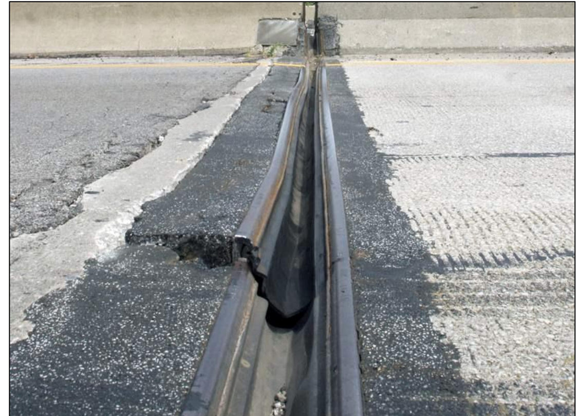
Bridge Expansion Joint with Offset on Both Sides of the Joint ( www.toledoblade.com/local/2011/07/08/Defective-bridge-expansion-joint-causes-I-75-delays.html )
