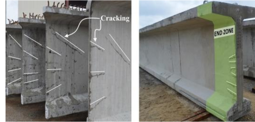
Examples of End Region Cracking (Ronanki et al. 2017)
