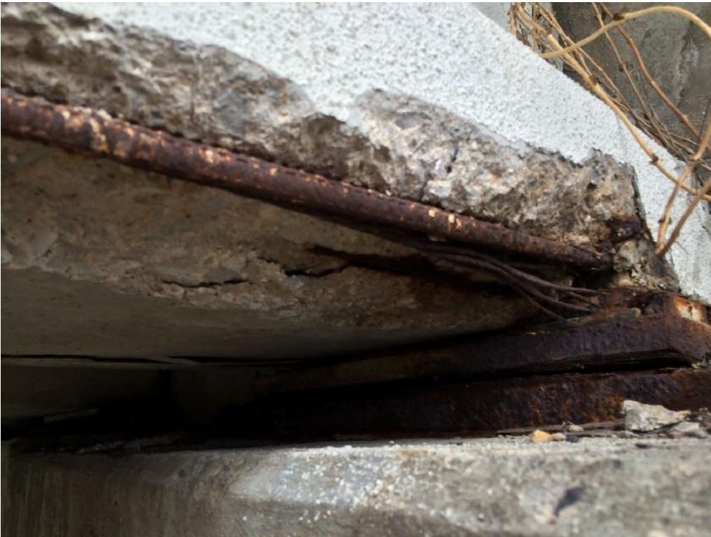
Spalling Along End Region Reinforcement in In-Service Prestressed Concrete Girder (Photo by Royce Floyd)
