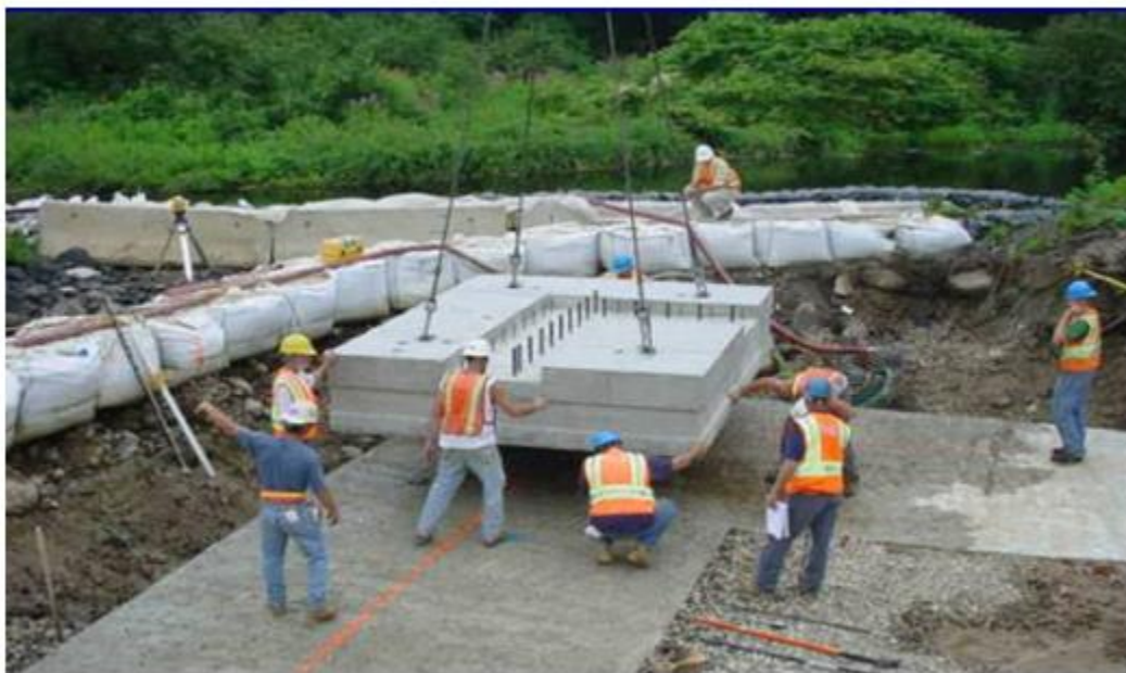
Figure 3 Installation of a precast concrete footing with grouted shear connection on concrete sub-footing [1]
