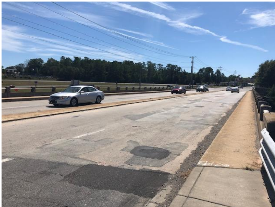
US 21 over I-20 – Columbia, SC - Existing Bridge Deck in Very Poor Condition – Fast Track Hydrodemolition and VESLMC Overlays were selected by the SCDOT to structurally repair the deck for 25 + years.
