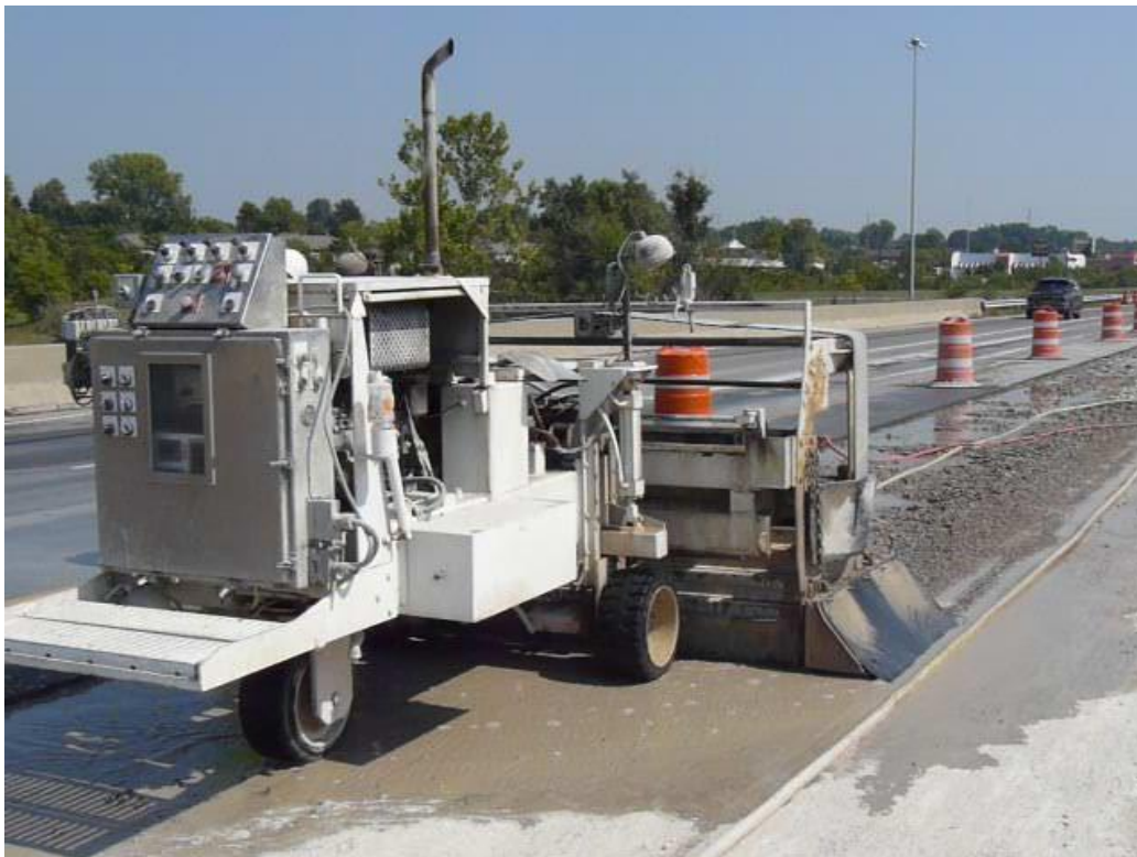
Hydrodemolition Robot performing Bridge Deck Surface Preparation on a weekend project next to live traffic
