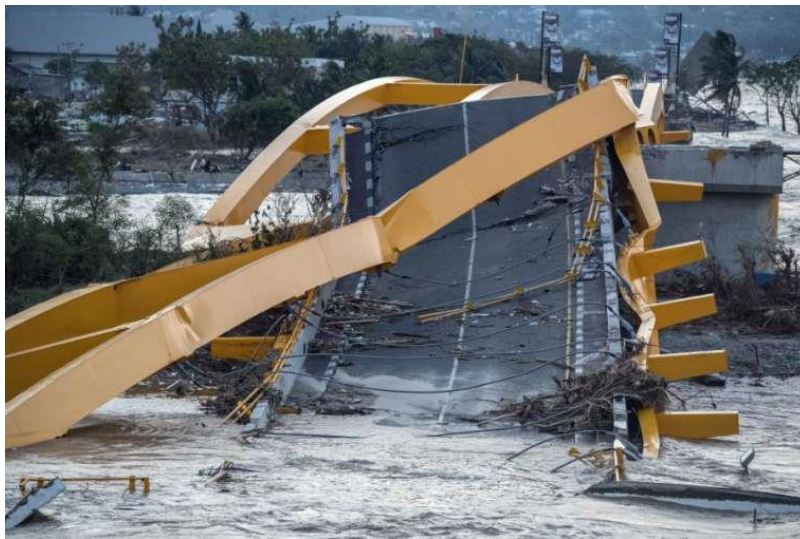
Figure 1. Ponulele Bridge Destroyed by 2018 Tsunami
