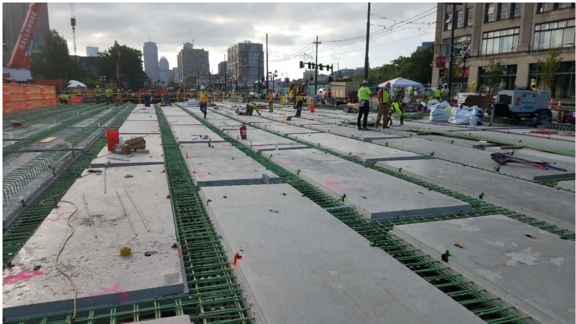
Precast Concrete Full-depth Deck Panels – Longitudinal Configuration Commonwealth Avenue Bridge Project, MassDOT
